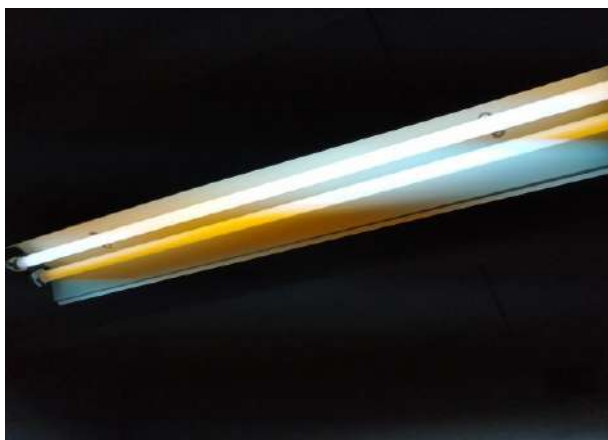
Figure 2.8: FLT lighting/illumination system
