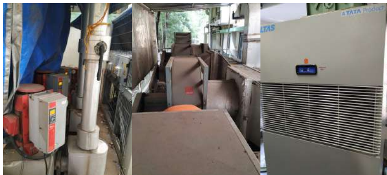
Figure 2.7: Refrigeration and air conditioning equipment
