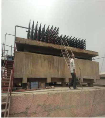
Figure 3.8: Atmospheric condenser unit for ammonia compressors
