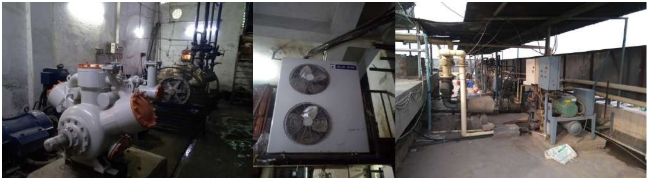
Figure 3.7: Common refrigeration system (L-R) Reciprocating ammonia compressor, scroll compressor, screw compressor
