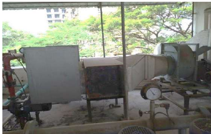
Figure 2.3: Treated fresh air fan unit
